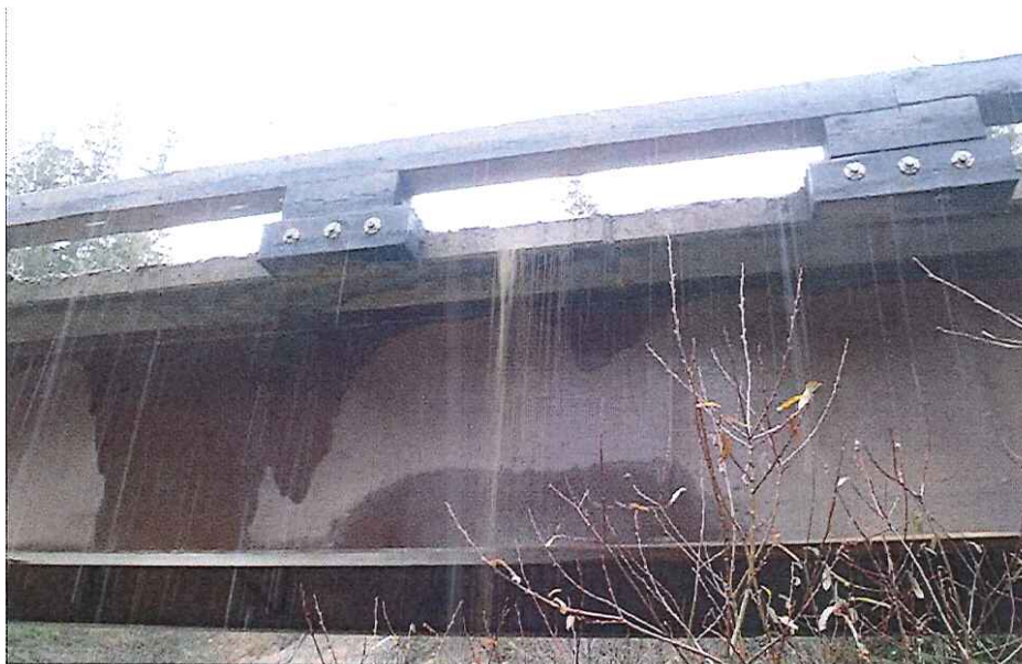
CK2306 Road drainage off deck into creek from...
